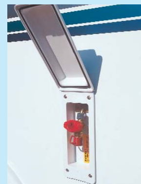
External gas BBQ point.
