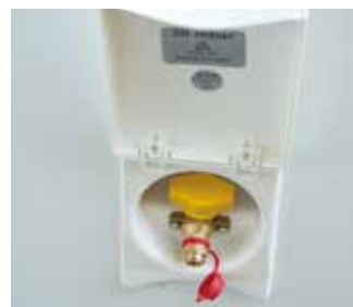
The barbecue point enables you to connect your barbecue directly to your caravan's gas
